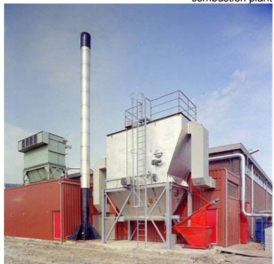
Figure 5.11 An electrostatic filter installed at a biomass combustion plant
