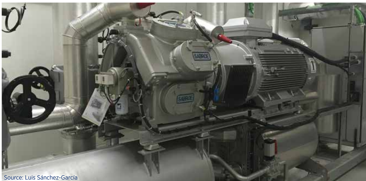
Photograph 3. Compression heat pump supplying a district heating system in Denmark
