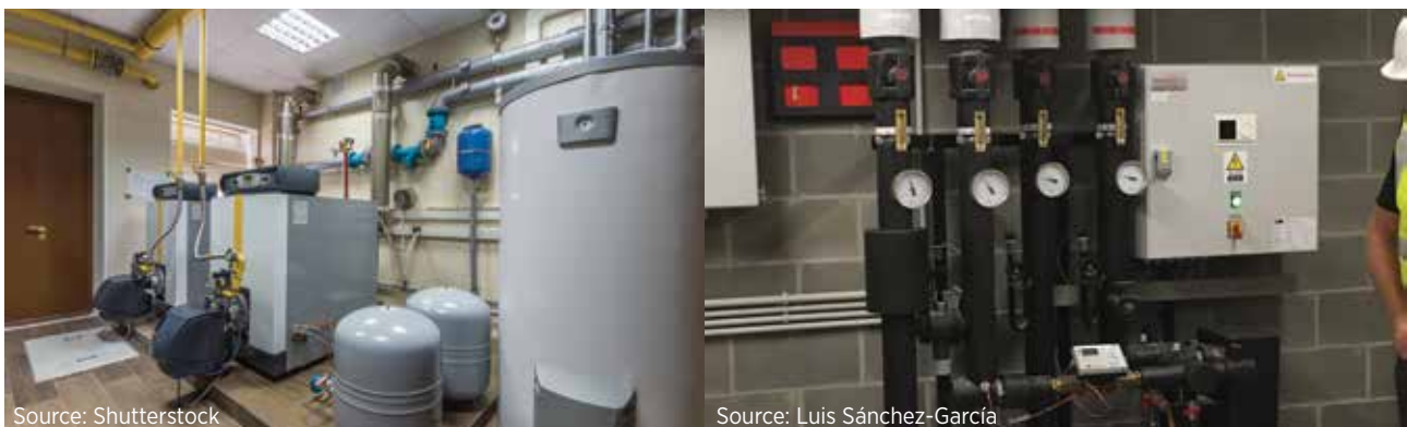
Photograph 5. Gas boilers in a gas boiler room (left) and a substation in a building in Belgium (right)
