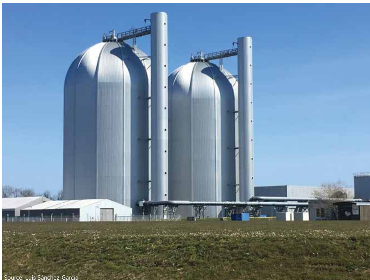
Photograph 4. Thermal heat storage (44 000 m 3 ) at Avedøre Kraftværket in Copenhagen (Denmark)
