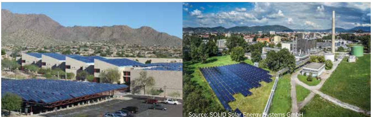
Photograph 7. Solar district cooling plant, Scottsdale, Arizona (United States) (left) and part of the Fernheizwerk collector field, Graz (Austria) (right)
